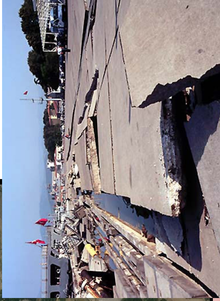
August 1999 Izmit-Turkey Earthquake Main pier and seawall of Gölcük Naval NIIGATA - JAPON 1964
