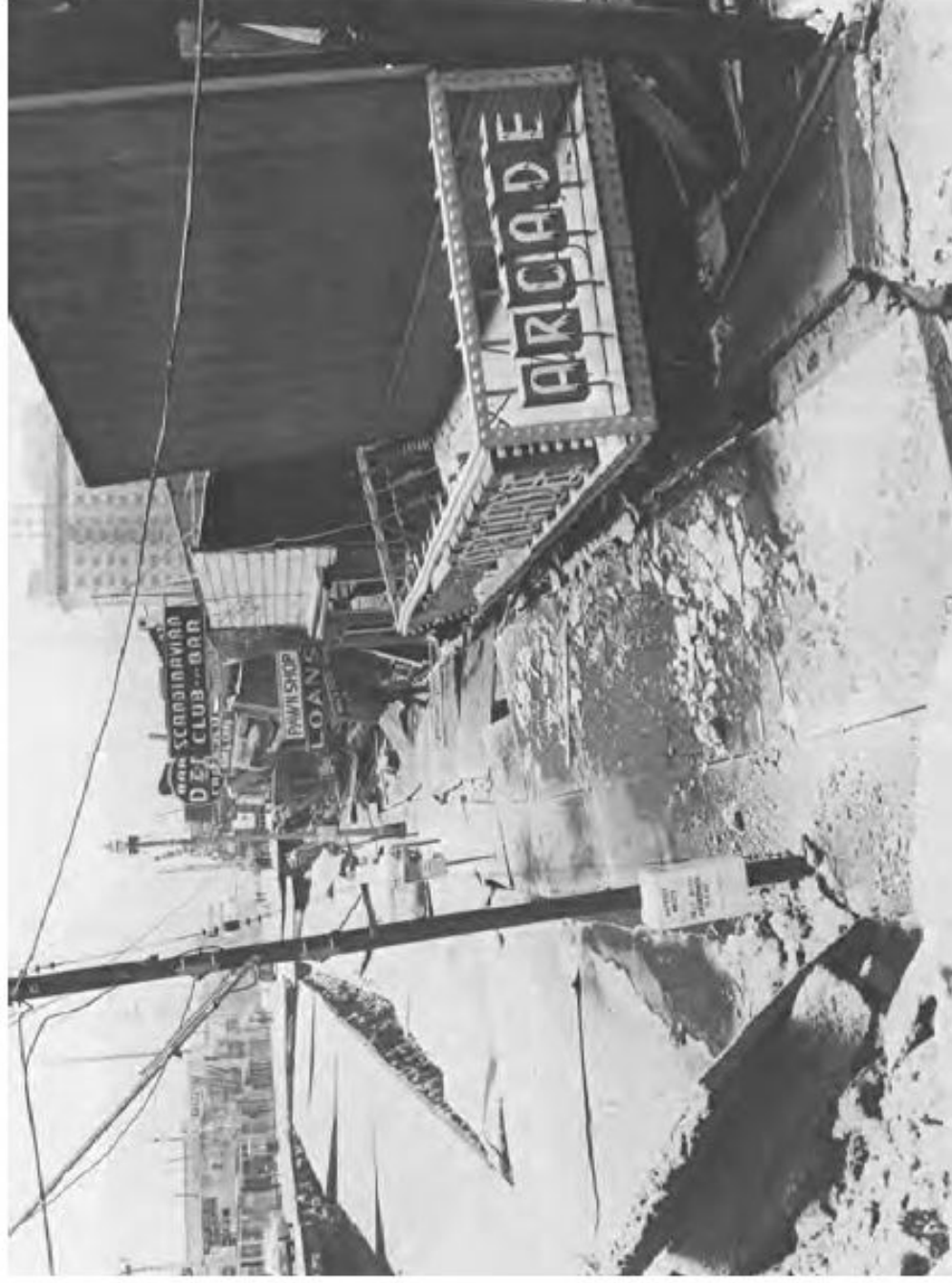
Figure 124. Ground failure along Fourth Avenue, Anchorage after the 1964 Prince William Sound, Alaska earthquake (photo: W. Hansen).
