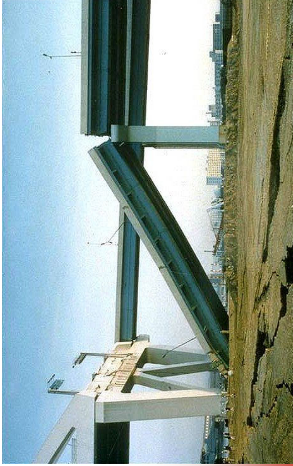
Nishinomia Bridge 1995 Kobe earthquake, Japan
